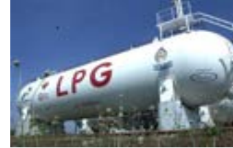
LPG Terminal & Bulk Clearance
